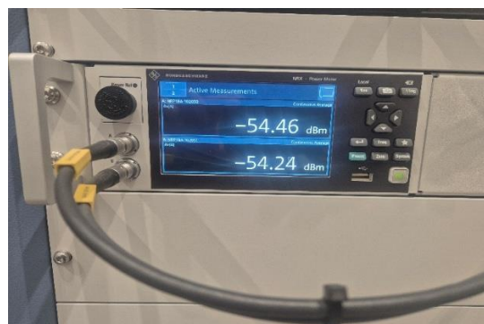
Figure 2. NRX power meter
