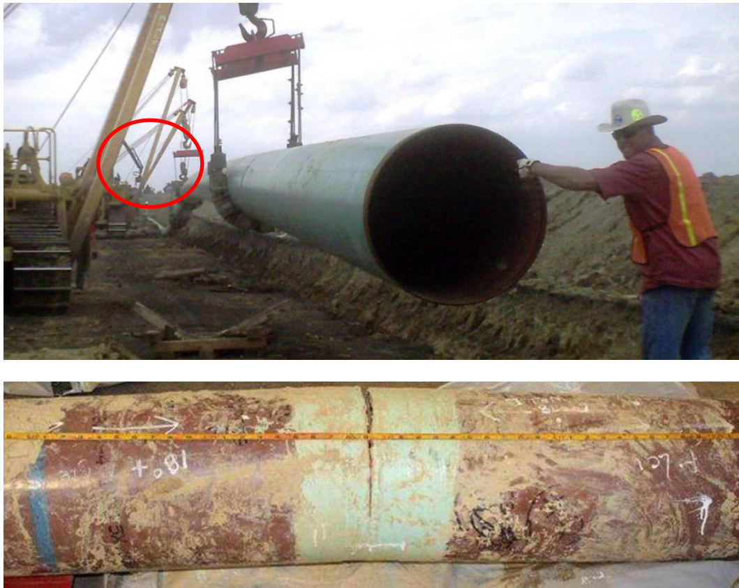
Figure 6. Above: Pipeline laying (Lee); Below: Girth weld crack caused by different pipe and ditch profiles (Bruce, 2017)
