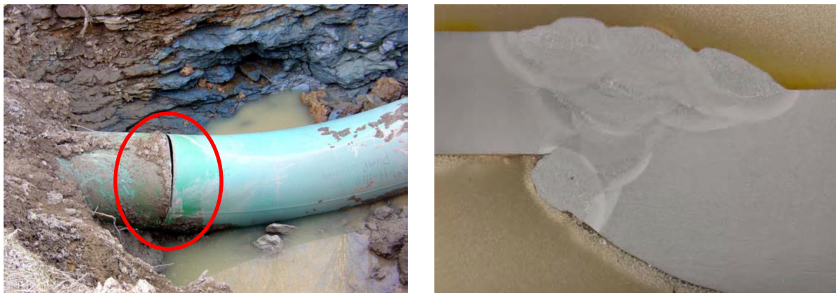
Figure 7. Connection of different pipeline section with different shape and wall thickness (Lee)
