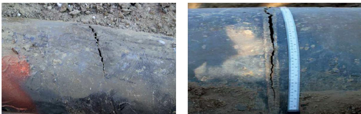
Figure 11. Examples of stress corrosion cracking (Chua, Alleyne & Calva, 2017)
