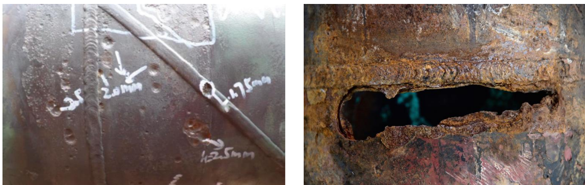
Figure 9. Corrosion defects near and on pipeline welded joints (Feng, 2017; Anon4)
