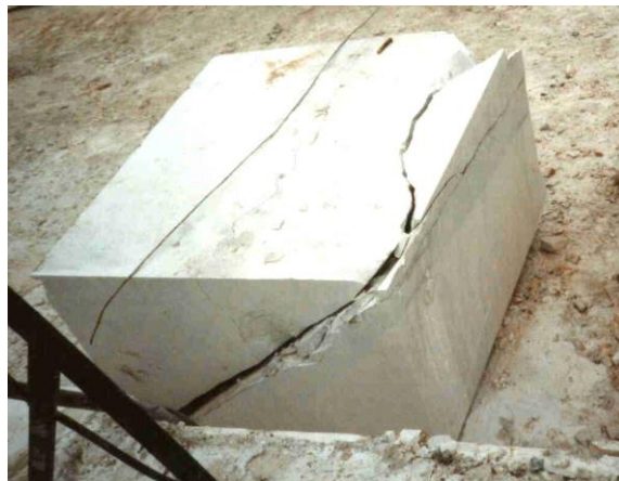
Figure 11. Fragmentation of a block due to cracks.
